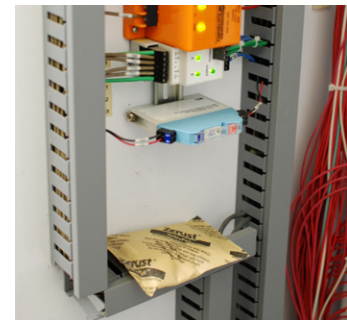
ZERUST® ActivPak® protects expensive controllers in a panel inside of a wastewater treatment plant.
