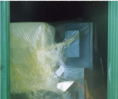
An electrical box protected internally by ZERUST® ICT® Vapor Capsules and externally by ZERUST® ICT®510-C Film.
